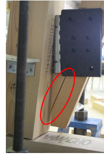
Picture 5: Split on the end of brace
